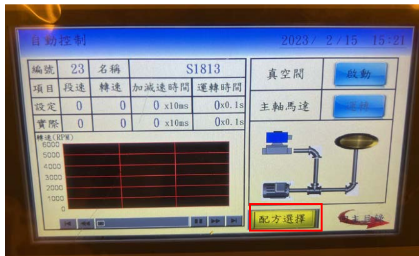
Figure 6 Automatic Control Interface
